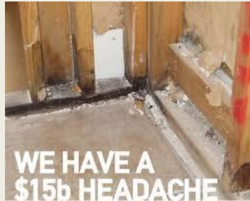
Leaky homes, NZ
